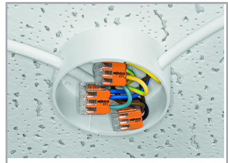
Lighting distribution in ceiling canopy
